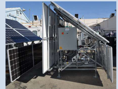
VariSun Solar Vapor Extraction Systems
